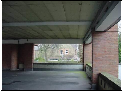
Ground floor rear parking area – first floor concrete frame and floor slabs visible
