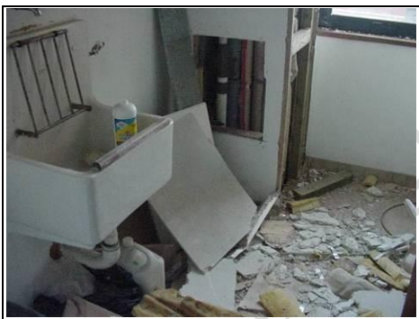
Service cupboard where core samples have been taken at ground floor, first floor and second floor
