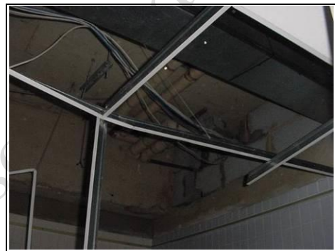
Ceiling down in gents toilets
