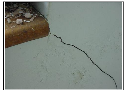
Close up of cracking
